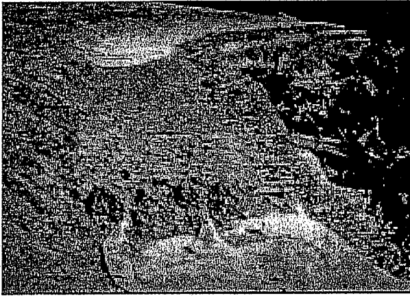
Figure 8.45: Partially installed vegetated geogrid. Installed above the toe to stabilize high bank.
