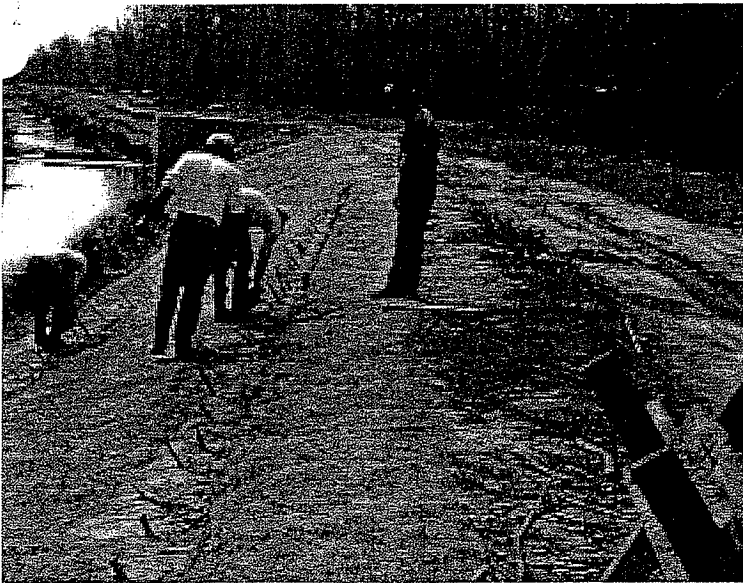
Figure 6.6: Contractor team. Contractors can assist in performing tasks that might be involved in restoration such as installing bank stabilization measures.
